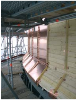
COUPOLE de l'observatoire de Meudon et sa nouvelle couverture. Dome of the Meudon observatory and its new roof.
